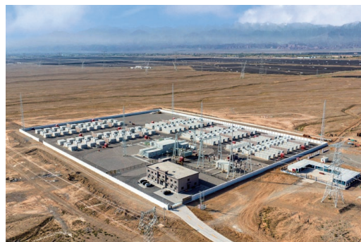
A location in Gansu: 1000MWh
